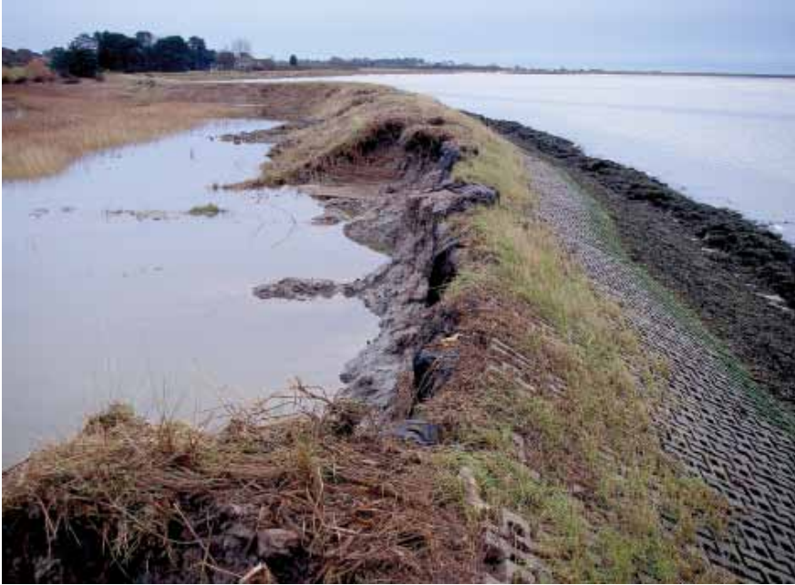
Damage to rear of river wall following December 2013 surge. Photo Andrew Hawes
