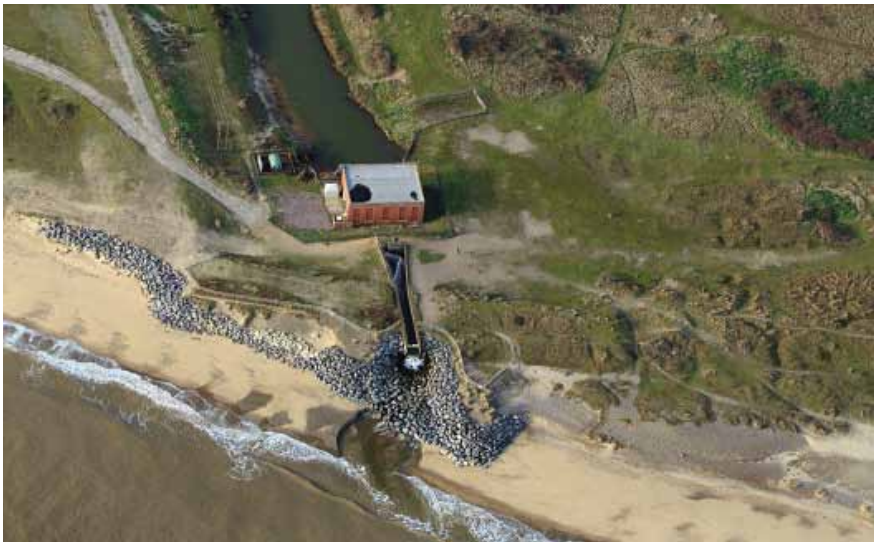
Benacre Sluice pumping station, rock armour visible on the seaward side. © Mike Page
