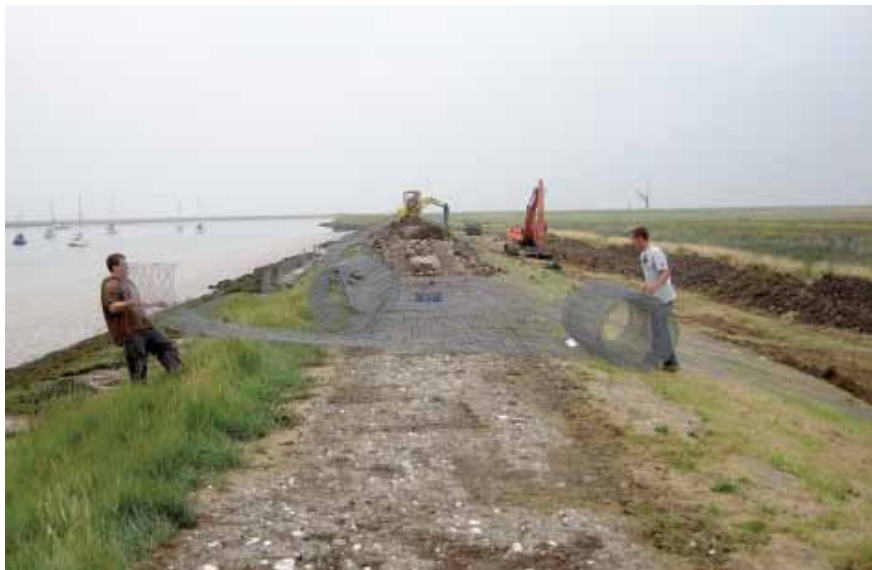
Trial river wall design at Orford, 2011. The wall height has been built up and the wall has been widened on the landward side to avoid breaching if overtopping occurs. Photo Amanda Bettinson
